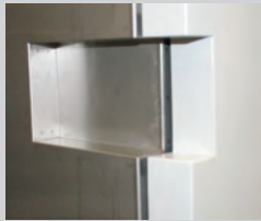
Notch-type access port in door
